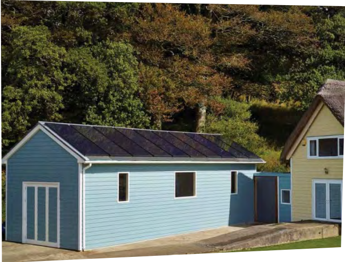
Eight solar panels and two solar thermal panels have been installed on the roof of this building in Cornwall. The panels are identical in size and colour, enabling an effortless combination of different forms of power generation.
