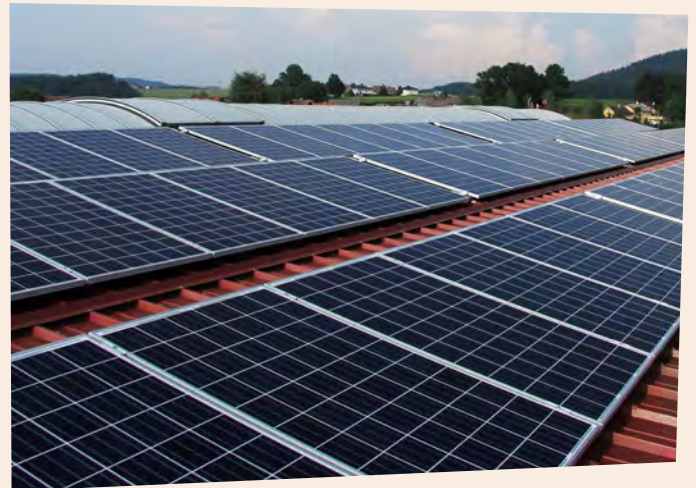
Polycrystalline solar PV with aluminium frames.
