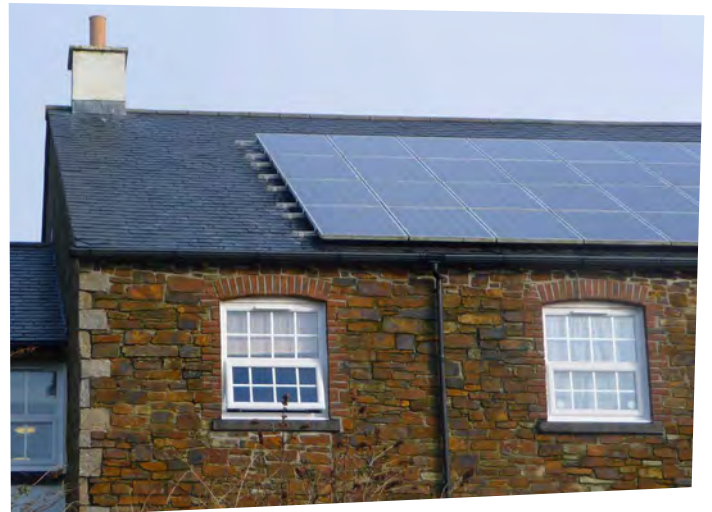
Example of a mounting rail protruding more than necessary.
