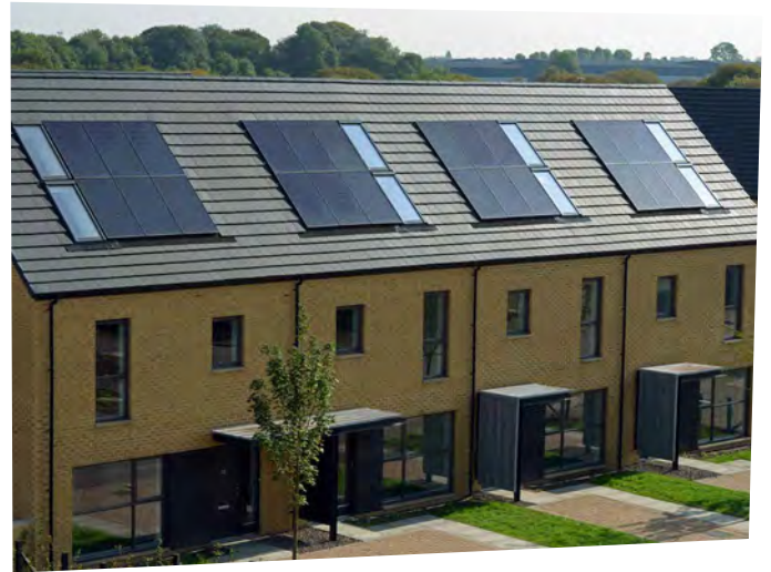
BIPV installation demonstrating good colour match of panels and roofing material at the Commonwealth Games Athletes' Village, Glasgow (see the case studies section).
