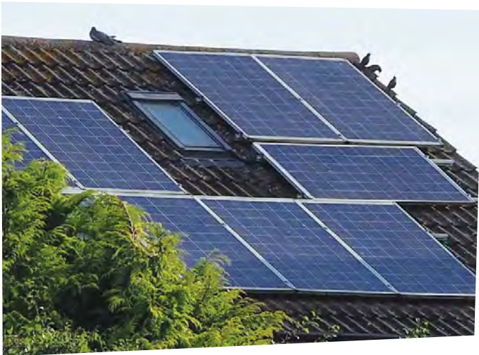
Non-symmetrically installed BAPV: panels are positioned in landscape and portrait format, panel edges are not always aligned and rails are protruding in an inconsistent manner.
