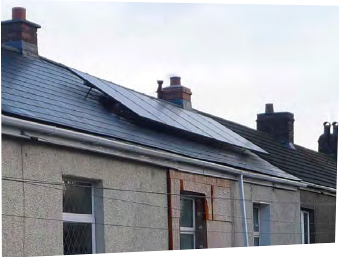
BAPV installation with a larger than necessary mounting system profile due to a high roof hook.
