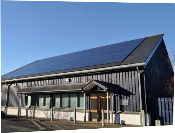
The Dyfi Eco Business Park shows BAPV with black anodised frames on a slate roof, where the panel colour is closely matched to the colour of the slate (see the case studies section).
