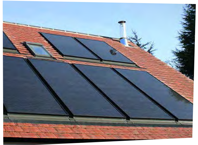
BIPV system with high degree of symmetry, achieved through consideration of roof furniture and installing all elements in portrait format.
